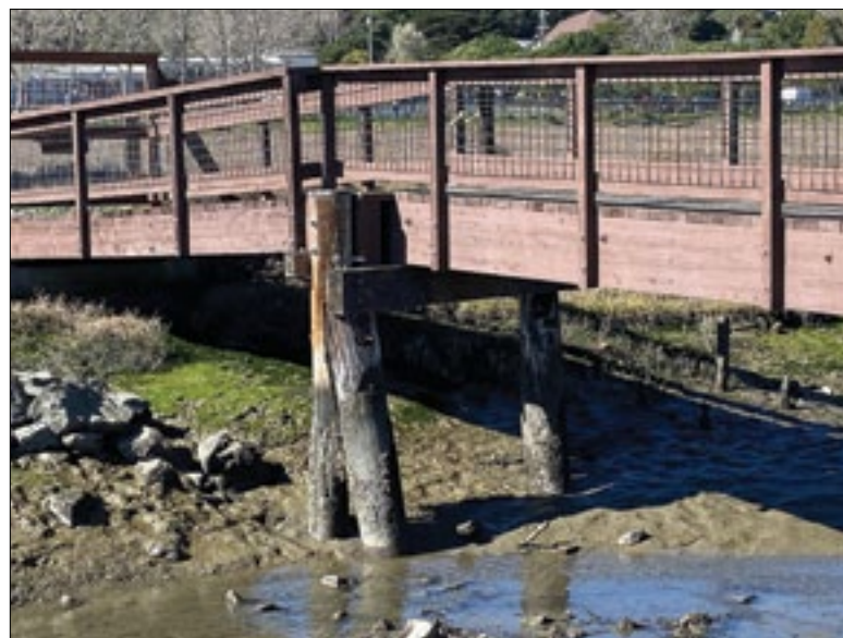
Signs of deterioration can be seen on the footbridge connecting a bayfront walking route between Tiburon and Strawberry that has been closed since late October after an engineer's report determined it was in need of repair.
